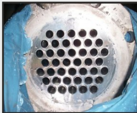
Gascooler gas pipings
